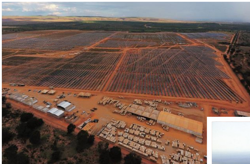
UFV de 185 MWp, Pirapora (MG).
